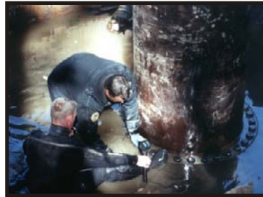
ABOVE: DIVERS INSTALLING MANHOLE ACCESS RISER (right in green) AS FINAL STAGE TO JOINT REPAIR AND PIPE ACCESS POINT
